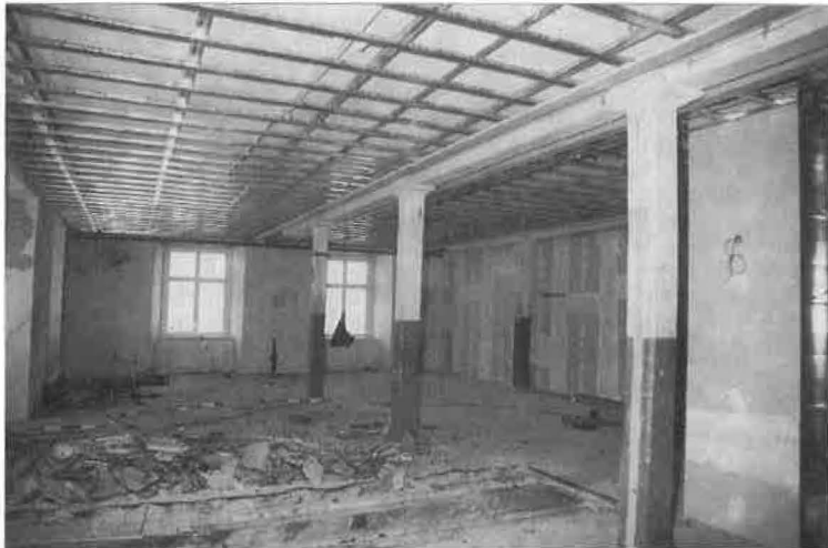
Figure 11: Reno- vating the former Lünensee factory – metal sub- structure for gypsum plaster- board ceiling
