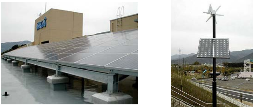
Figure 7: Energy saving equipments (KAMPO new facility policy for environment)
