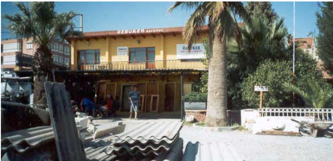
Figure 4. Front view of the double storied office building in the demolition contractor's yard in Buca.
