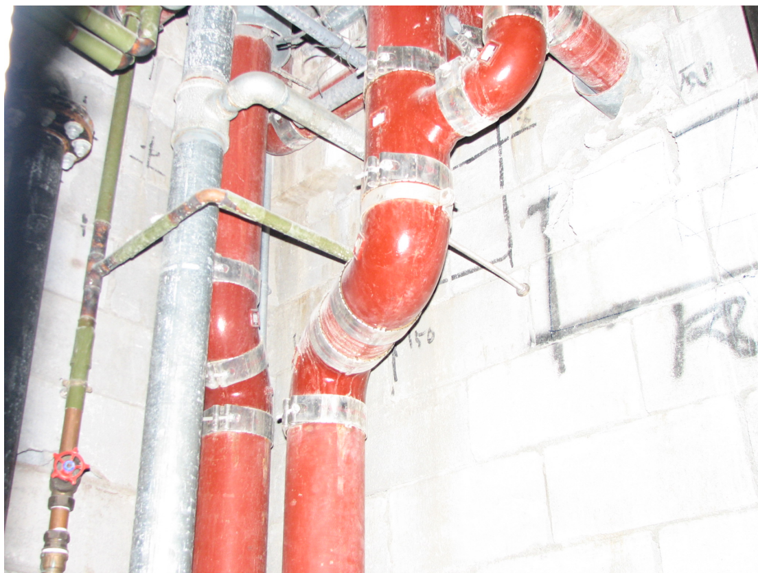
Figure 2 Unnecessary bendings along the vertical drainage stack
