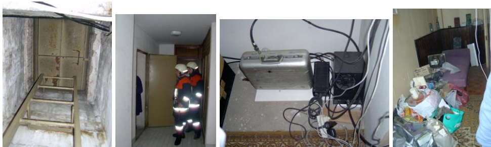
Figure 8-11: Locked staircase ventilation opening, apartment door in hall end, behind escape door, dangerous wiring and flammable materials in fire escape staircase
