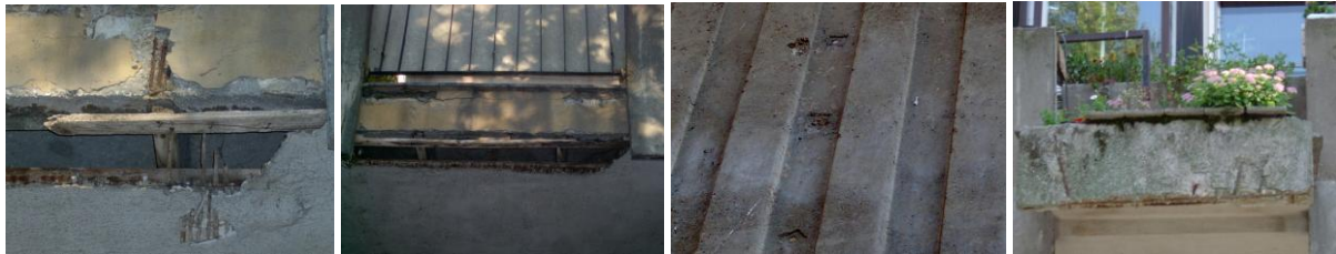
Figure 4. Damaged surface layer of prefabricated elements: corrosion of concrete and steel bars
