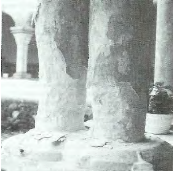
a) Loss of material in columns (14)
