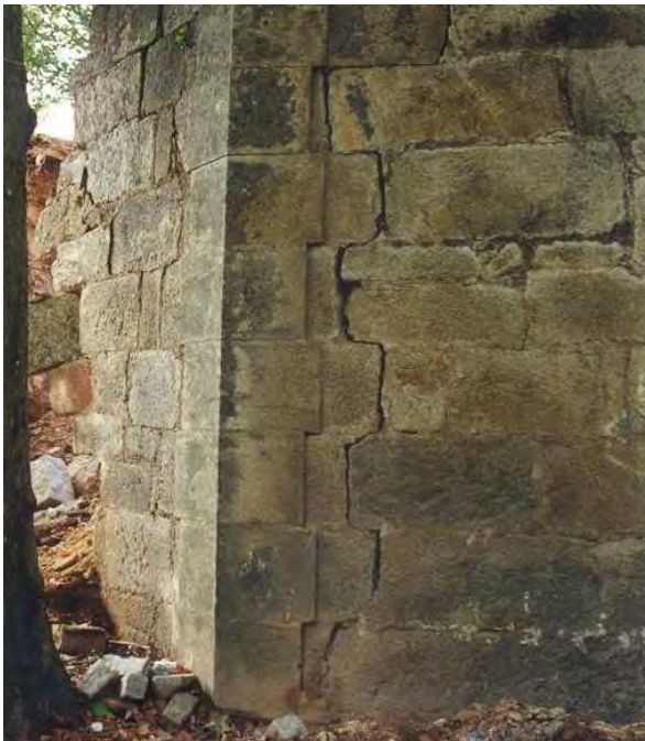
Figure 5: Damage in walls due to earth pressure (21)
