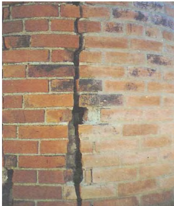
Figure 8: Vertical cracking in a masonry chimney (21)
