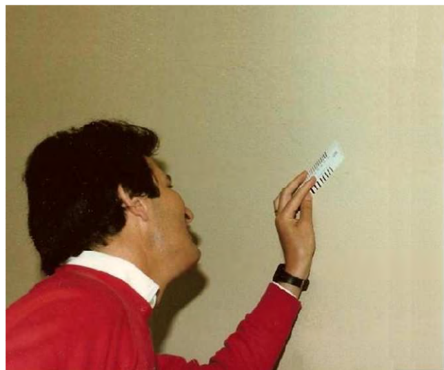
Figure 17: Ruler measuring the width of cracks in walls (21)
