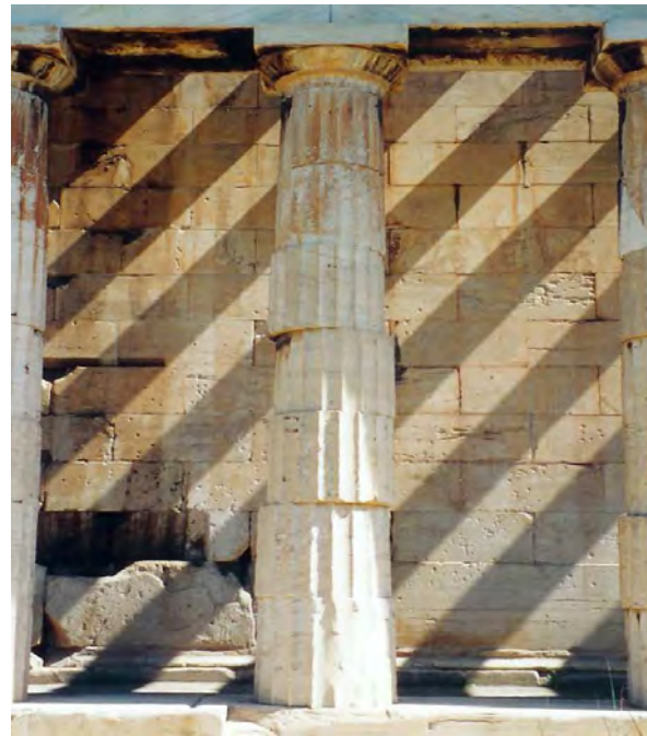
Figure 6: Damage in column due to earthquakes (21)
