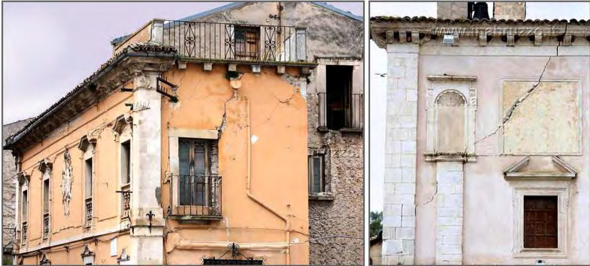
Figure 4: Damage in walls due to earthquakes (40)
