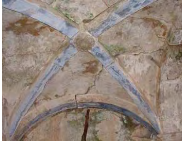
Figure 7: Cracks in a masonry vault (24)
