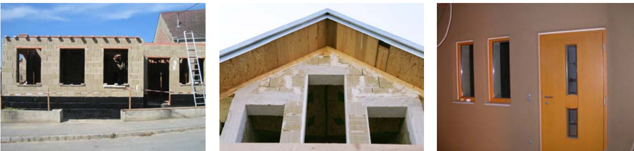
Figure 5: Fired lintel element, leveling concrete course around wall opening and airtight connection of windows and doors for Passive House Standard.
