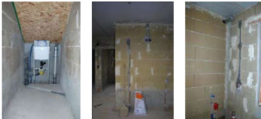
Figure 7: Water pipes are mainly led into the floor. Installation lines in the unfired loam brick walls are not a problem.
