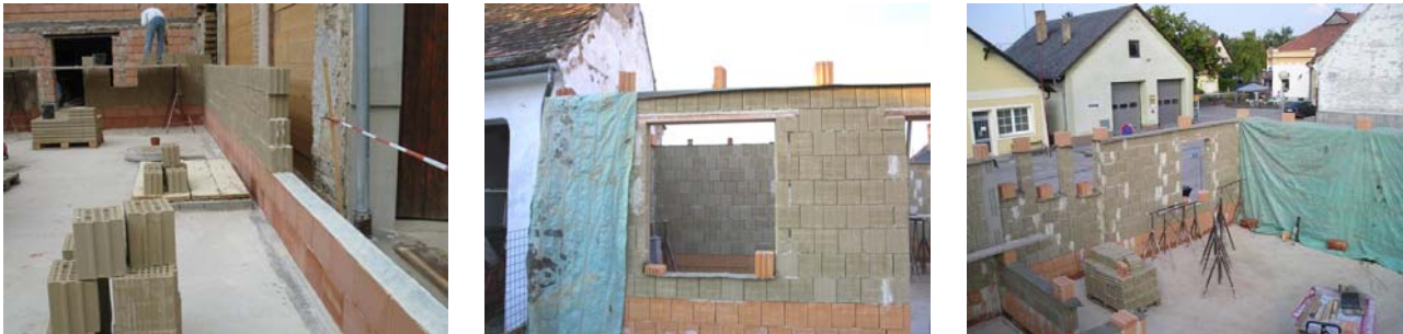
Figure 4: The first two layers were constructed with fired loam bricks. The last layer under the sills and top layers of the walls have been covered with a waterproof material to prevent water inside the brick perforation.
