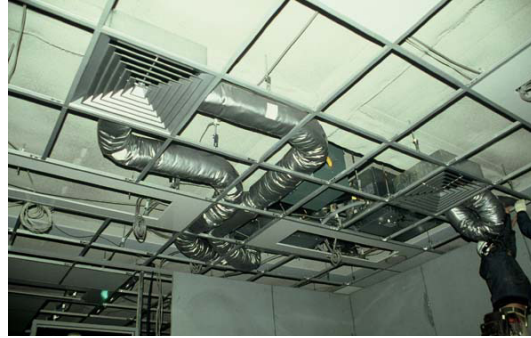
Figure 6. Ceiling and mechanical equipment
