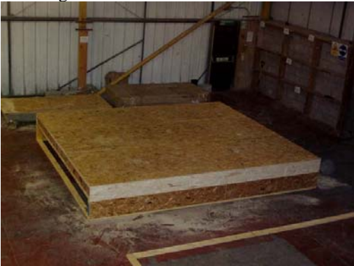
(d) A floor, decked with OSB and supported along two edges, was completed.
