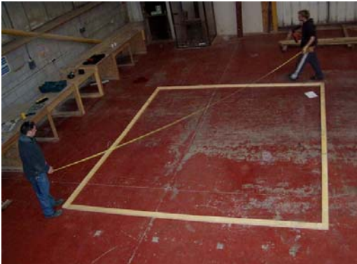
(a) A timber frame was fixed to the concrete floor using nails.
