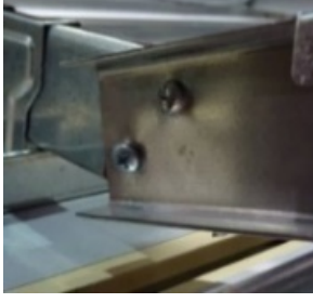
Photo 2: Damage at the joint. (No. 4)
