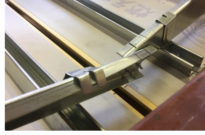
Photo 3: Lateral deformation of C-bar. (No. 6)
