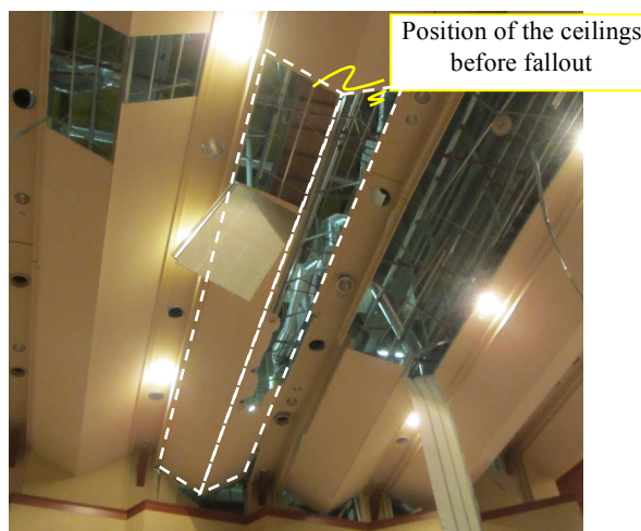
Photo 1: Earthquake damage on the ceiling of a hall with multiple slopes. (NILIM, et al. 2016)
