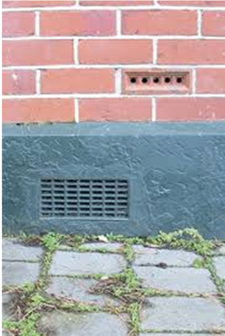
Fig 6: picture showing vented cavity wall (the red brick is a ‘cavity vent’) and sub-floor ventilation below it, painted grey. The inexperienced Energy Assessing Surveyor might mistake one for the other, and the consequences are outlined in figures 3 and 4 below. (W-Y-P Gledhill, 2005)
