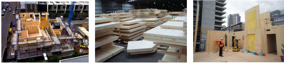
Figure 5 a, b and c: The 10-storey 'Forté' apartment building in Bourke Street, Melbourne Docklands, under construction (July 2012); CLT panels stored in a warehouse close to the site. (Source: C. Philpot, 2012; S. Lehmann, 2012)
