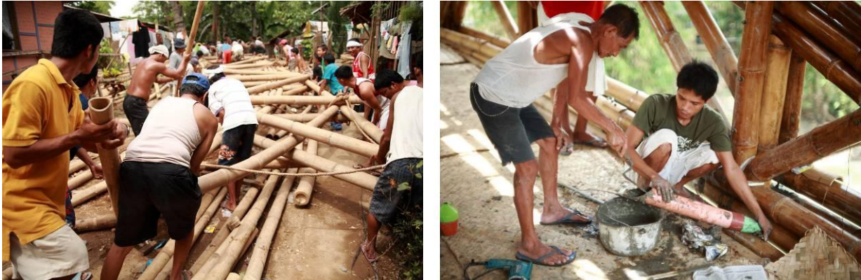
Figure 9 Men push a completed frame to the foundation (left), sand-cement mortar injection on main joints (right)
