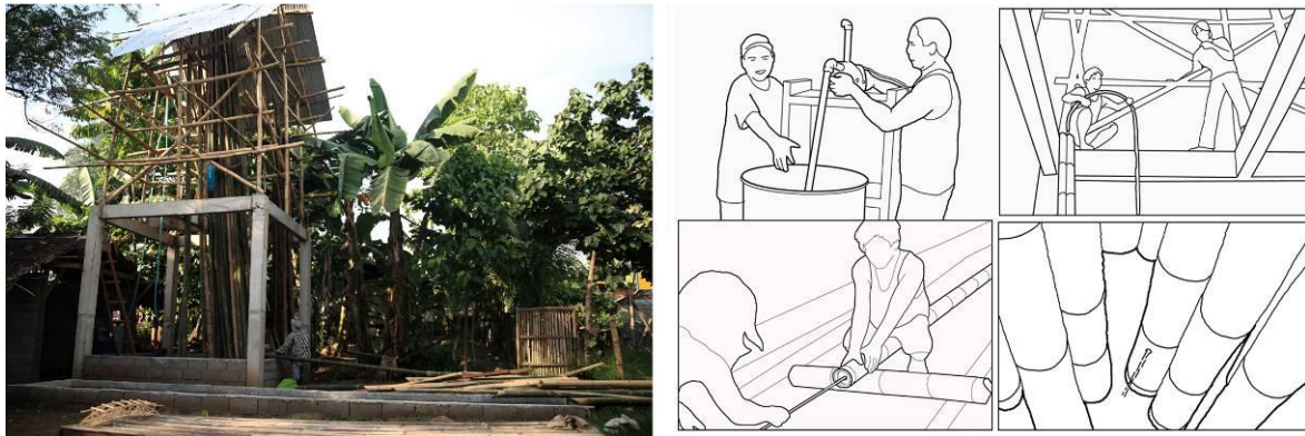
Figure 7 Vertical Soak Diffusion (VSD) plant adjacent to the bridge's site (left) and illustrations of the treatment process (right)
