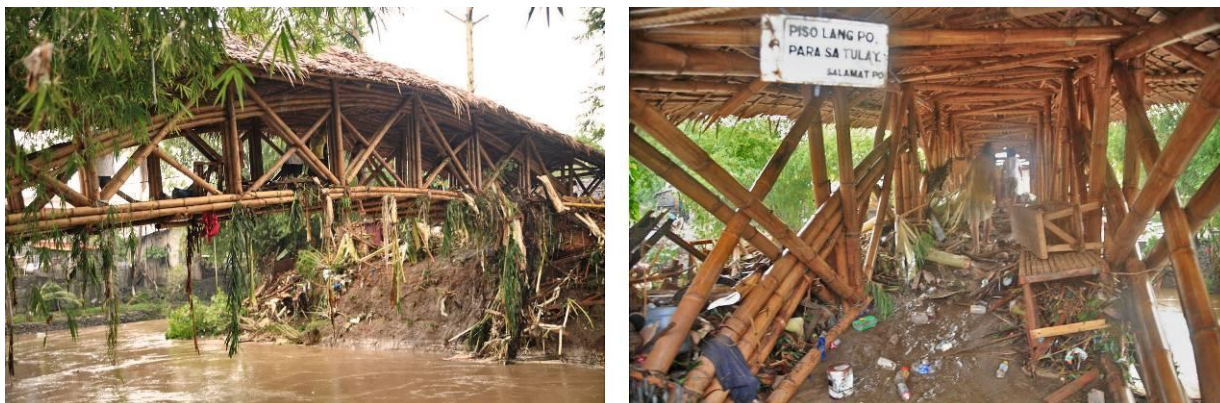
Figure 10 Debris brought by July 27 flash flood (left) engulfed the bridge (right), and the concrete floor which seamlessly connects the bridge to its foundation saves the bridge.
