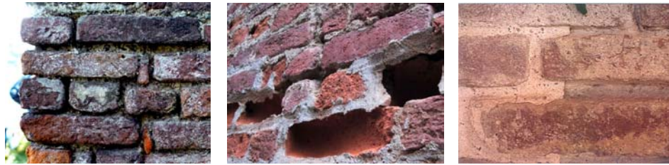
Figure 1. Efflorescence on bricks and loss of mortar joints before re-pointing; b) effect of incompatible pointing mortars in case of good adhesion and c) in case of bad adhesion.
