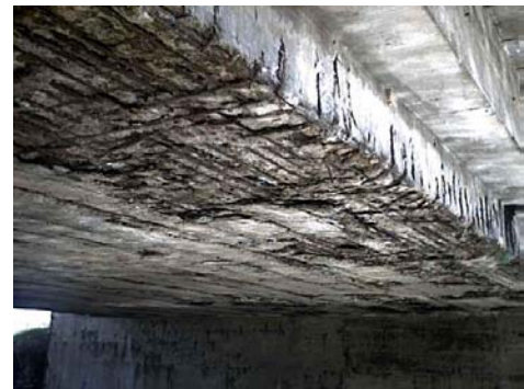
Figure 3. Conditions of the bridge before repair measures were taken.
