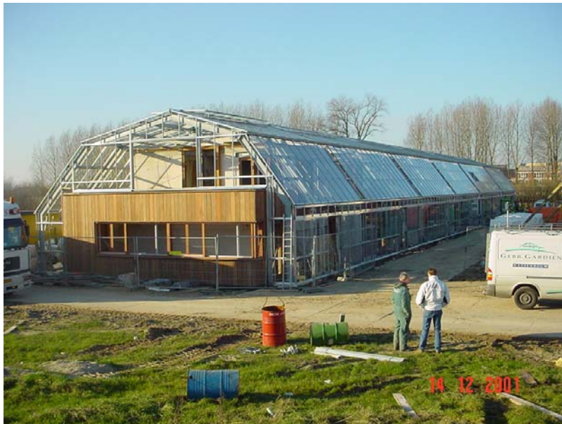
Fig 4 New row houses under a glass skin being built in Culemborg, Netherlands (2001)
