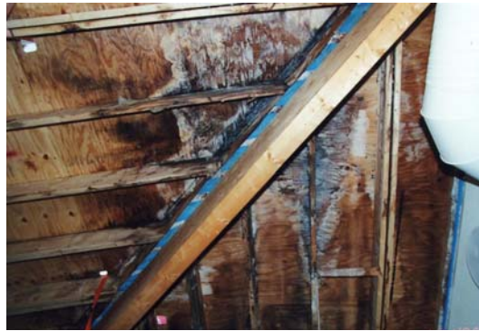
Figure 1. Deterioration of plywood in a sloped roof made with wood-based elements assembled in situ. Due to leaks in the joints between elements in the corners, humid air has penetrated into the construction, where it condensates on the cold surfaces above the insulation.
