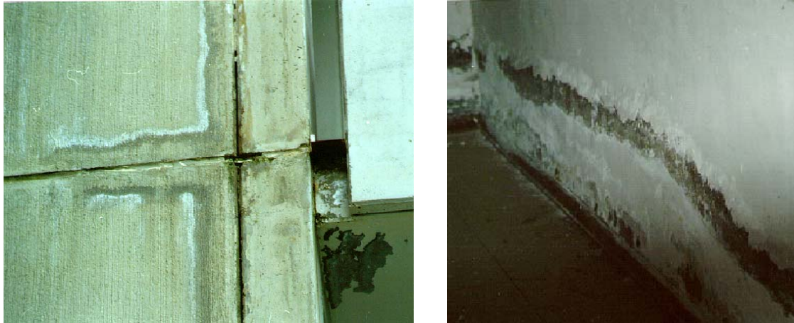
Figure 4. An example of the lack of attention in the carrying out and junction of single strata prefabricated panels. Some of them presents breaches and the most part of joints are not adequately sealed. It is inevitable in this way that there are leakings of water and infiltrations of air inside the habitable rooms, causing the creation of thermal bridges.
