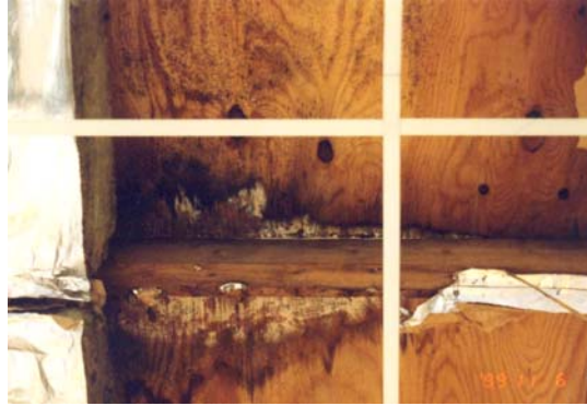
Figure 2. Leaks in the vapour barrier (as seen to the left) due to poor workmanship allow humid air to penetrate to this school roof, where it condensates and causes mould attack and dry rot.
