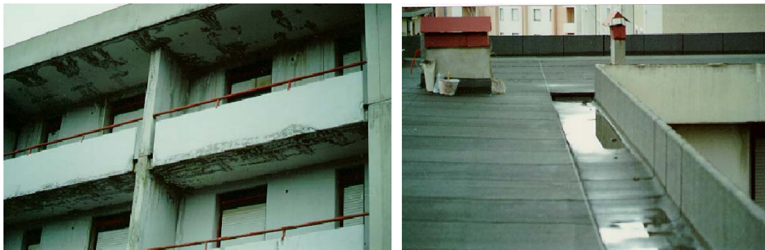
Figure 5. The wrong project of water piping and collecting system produces leakings of water caused by stagnation, cracks, lack of cohesion of concrete, stains on external surfaces.
