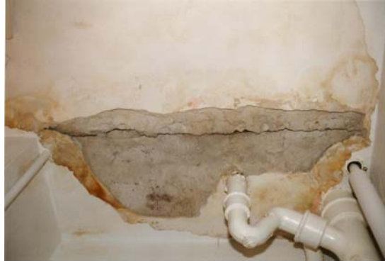
Figure 3. Penetration of water through a floor constructed with a solid steel profile with concrete. The penetration is caused by water entering cracks between an old and a new floor, because the floor gully was not replaced. The steel corrodes and expands causing the cracks to grow bigger, thereby accelerating the deterioration.
