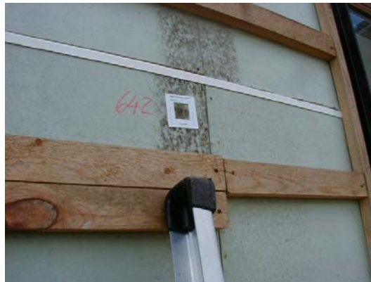
Figure 6. Façade with mould growth on wind barrier made with gypsum boards. Often mould growth in facades is due to water penetrating behind the cladding without being drained out (fast enough).
