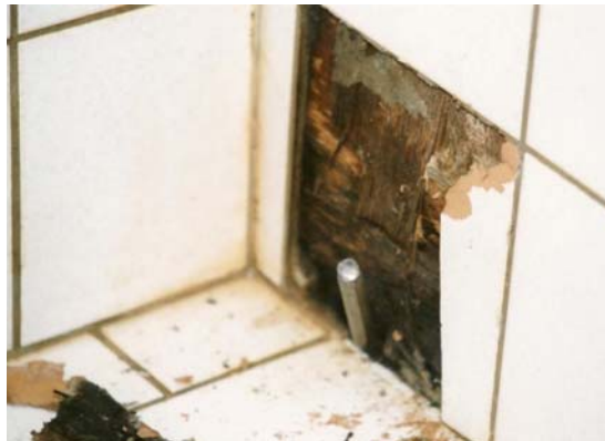
Figure 4. Deterioration of plywood wall and entire floor construction due to ceramic tiles applied directly on plywood - without watertight membrane. Besides the missing membrane the construction was too weak to resist dimensional changes in the plywood.
