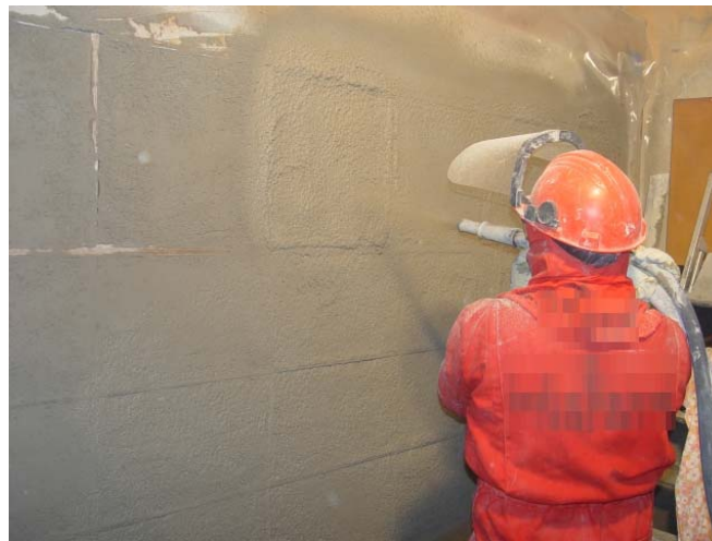
Figure 3. Application of the wet sprayed mortar (thickness 6 cm) takes place at the manufacturer.
