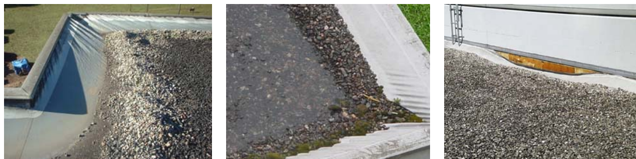
Figure 3. Examples of damage found on roofs with synthetic membranes.
