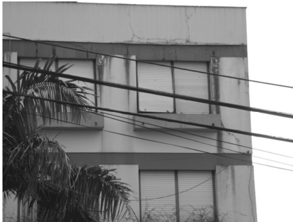
Figure 2. Roof covered with fibro cement with plate-bande presenting infiltration stains.
