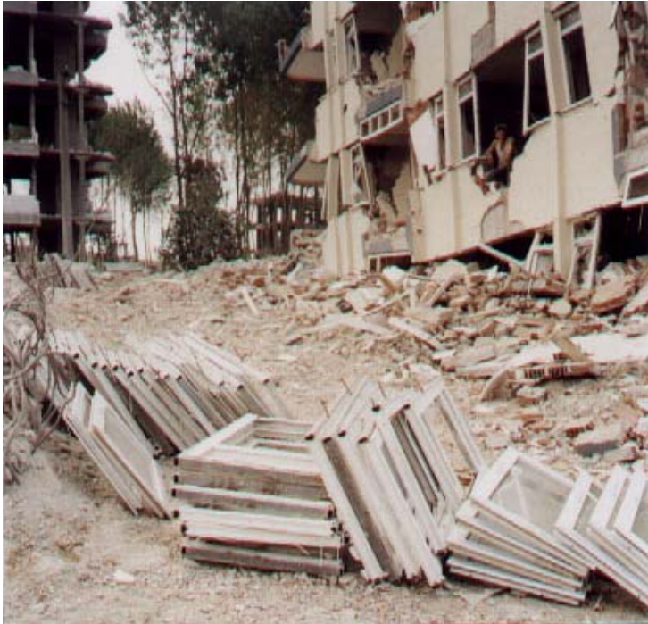
Figure 13: Rear view of the building in Figure 12 shows men working in this dangerously tilted structure to dismantle building components and fixtures; salvaged fenestration units are seen collected in the foreground [i].
