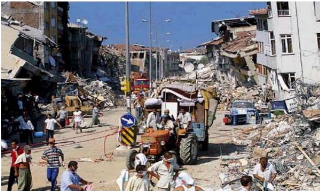
Figure 2: Another view of the main road, shown in Figure 1, after demolition work had started on the dangerously damaged buildings [iii].
