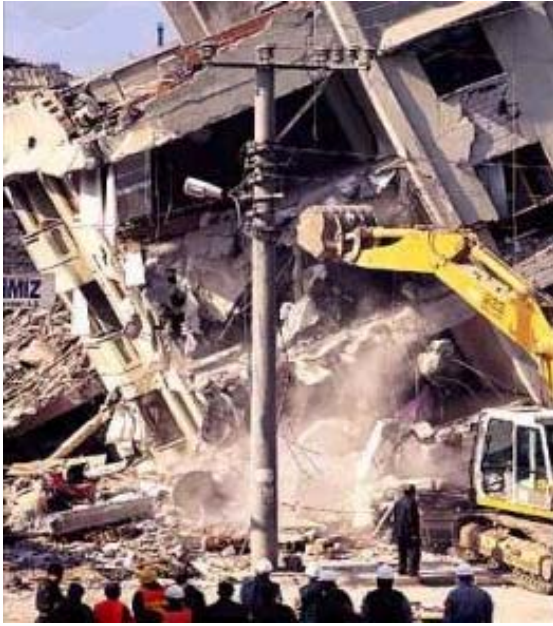
Figure 7: A semi-collapsed structure being pulled down in Adapazari [iii].
