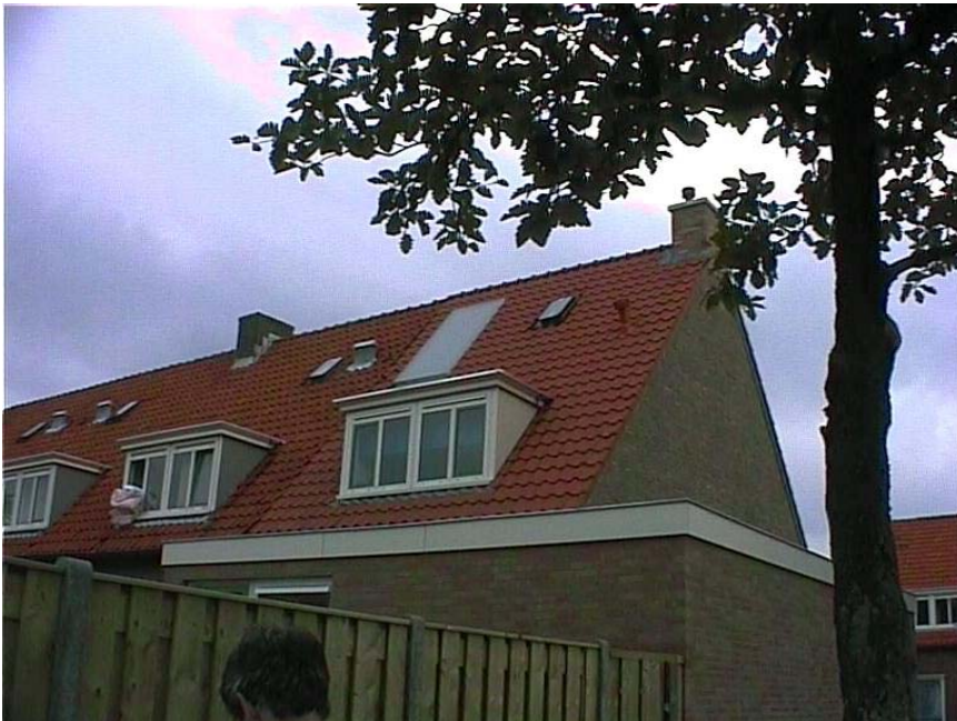
Figure 9 Renovated roof with PV panel
