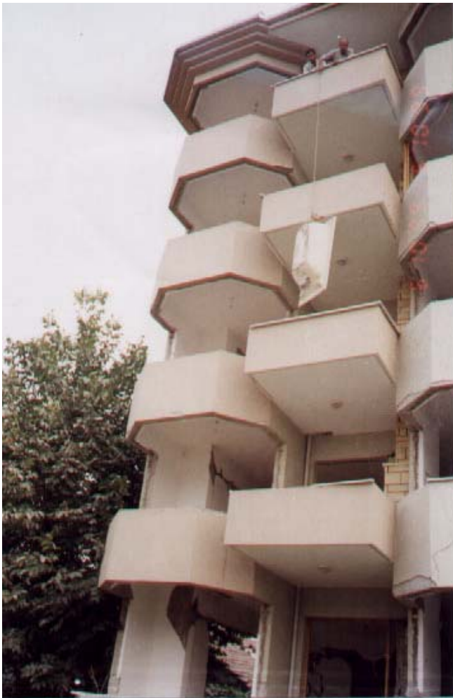
Figure 14: Deconstructing a severely damaged, newly constructed building in Golcuk: Bath tub being lowered from the 5th floor of the building whose ground floor had buckled under [i].
