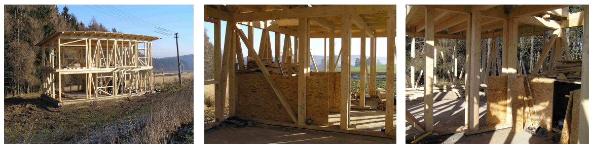
Fig. 1 Timber structure of the family house in Kozmice (12/2006). Two parallel diaphragm interior walls creating cavity for distribution of heating air will be built from prefabricated wall panels
