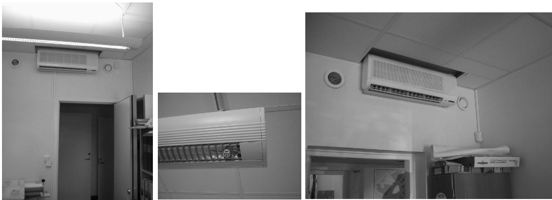
Figure 2: The test room installations. For the end-users' convenience the control of the heating fan coils and the lighting and their different combinations are in focus in the design and testing of forgiving technology.
