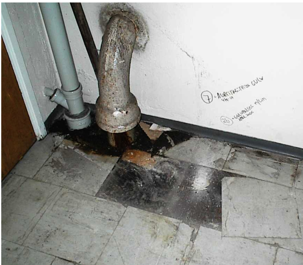
Figure 1 Picture of vinyl floor in the new administration building at the hospital (Rikshospitalet) in Oslo where samples were taken and analysed. The material under the vinyl tiles contained PCB in a concentration of 19.7 ppm.
