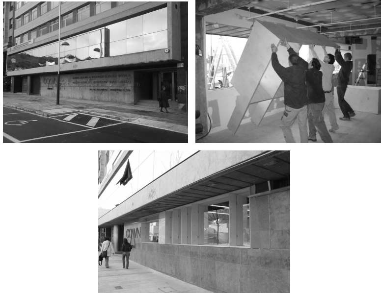
FIGURES 10,11,12: previous situation, process and final result in the Basque and Navarre Architect's Chamber, Bilbao. Project by Metak Arkitektura Tailerra .
