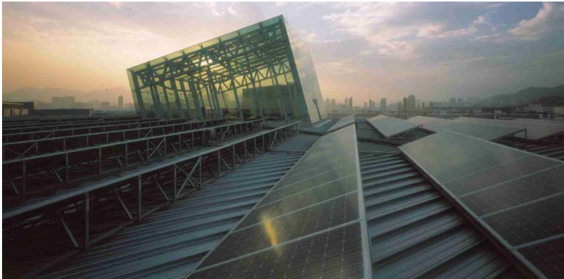
Fig. 3 PV panels & BIPV
