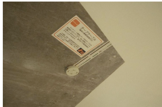
Figure 30 KSI electric wiring
